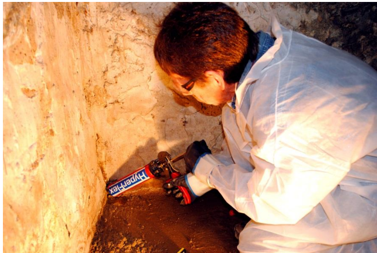
In this photograph, HyperFlex is being used to fill a void found on the other side of this very old farmhouse wall.
